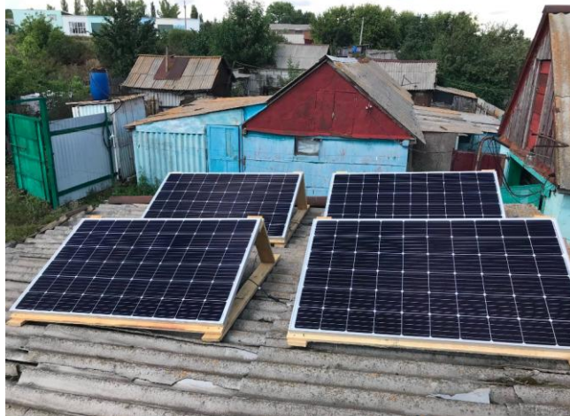
Figure 1 – Installed solar panels
