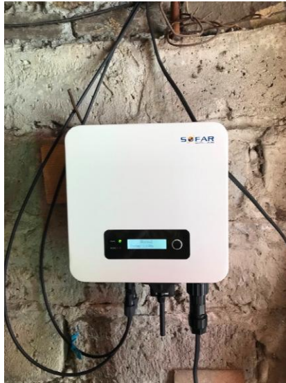
Figure 2 – Installed Sofar inverter
